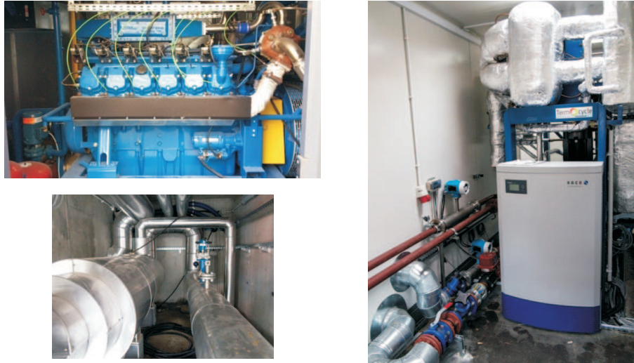
Figure 3: The combined gas/vapour (ORC) power plant: internal combustion engine from MAN (top left), heat recovery boiler (bottom left), 40 kW ORC system (right).
