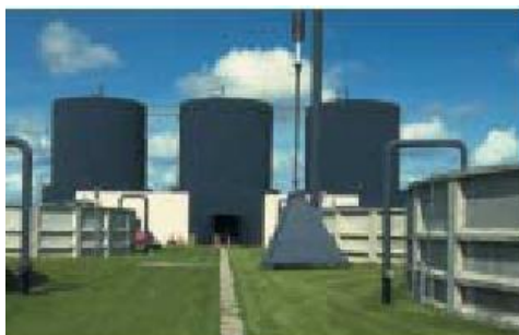
Large scale Danish biogas plant at Lemvig, noted as successful case study in IEA BioEnergy Report (2005)
