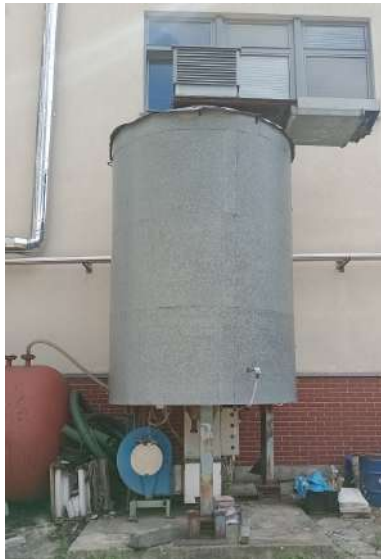
Fig. 13.6: Inlet with drying unit.
