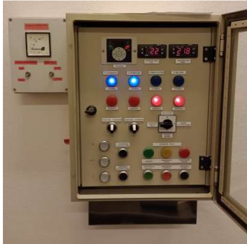
Fig. 13.26: Control panel in 'Ready-to-work' state.
