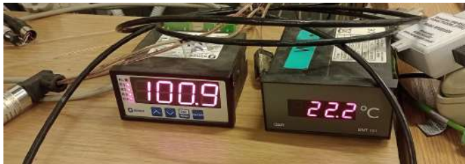
Fig. 13.27: Vacuum tanks pressure and stagnation temperature displays.
