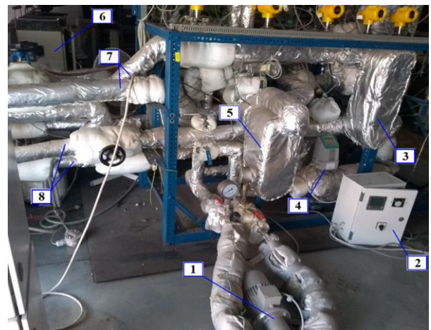
Fig. 3. Micro-ORC power plant test rig: 1 – pumping engine, 2 – frequency converter connected to the PE drive, 3 – evaporator, 4 – Coriolis mass flowmeter, 5 – condenser, 6 – control and regulation module for the induction heater, 7 – heating cycle piping, 8 – cooling cycle piping.
